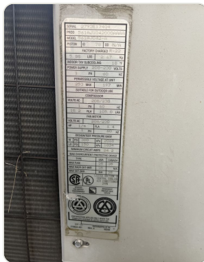
data plate · older unit — even a faded label tells us age and refrigerant.
