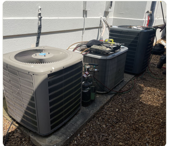
on site • arriving with the right parts is the whole point of showing us the unit first.
