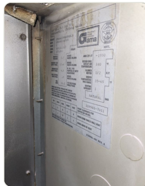
data plate · furnace — inside the front panel; flashlight on.
